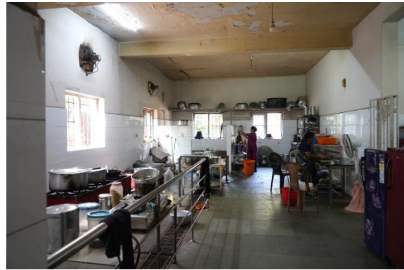
DETERIORATIONS IN THE OVERALL STRUCTURE
